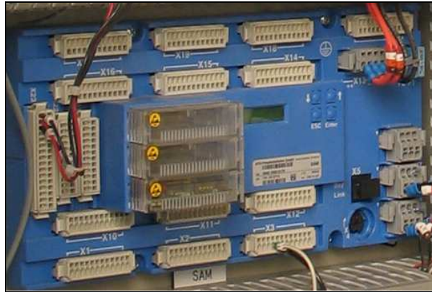
SAM module mounted in the customer panel
